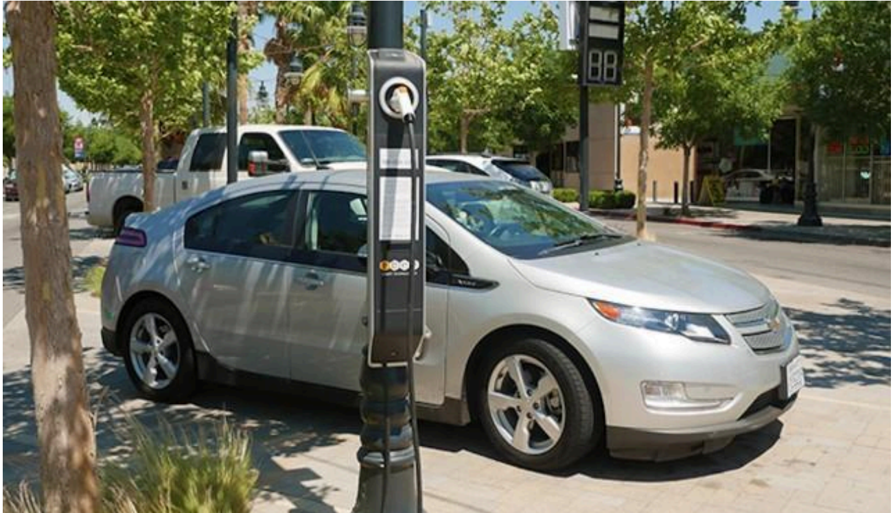
Ebee Streetlight Charging Station in Lancaster, Calif. (Photo courtesy of Green Car Reports)
